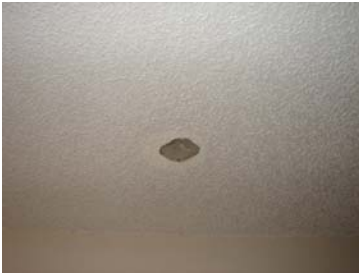
Missing Light at Front Door
