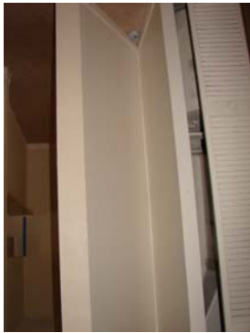
Missing Closet Door
