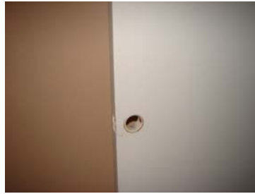
Missing Door Handle
