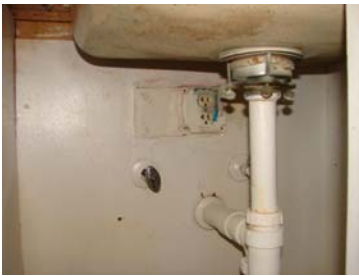
Missing Hot Water Line
