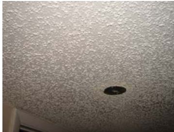
Missing Light in Hallway
