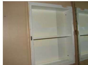
Missing Medicine Cabinet Door
