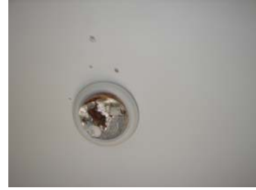
Missing Smoke Detector
