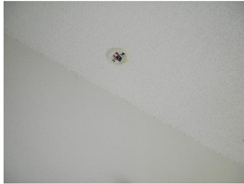
14. Missing Smoke Detector
