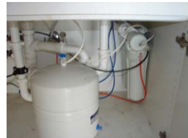
Well Components Under Kitchen Sink
