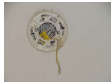
Missing Smoke Detector
